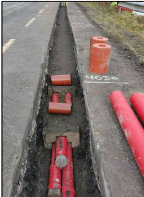
Plate 2-1 110Kv Cable Trench View
